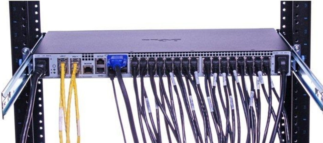
Figure 7: Two Post Rack: System and Cables Installed
